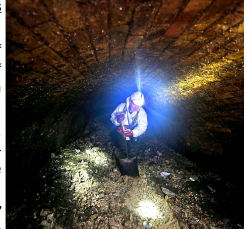
A Thames Water sewer supervisor in a sewer in London in 2014. The mass that the company has found to the east of the financial district is expected to take three weeks to remove using hand tools and water jets. Credit Adrian Dennis/Agence France-Presse
